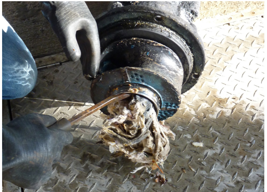
Wipes being removed at a Kitsap County pump station
