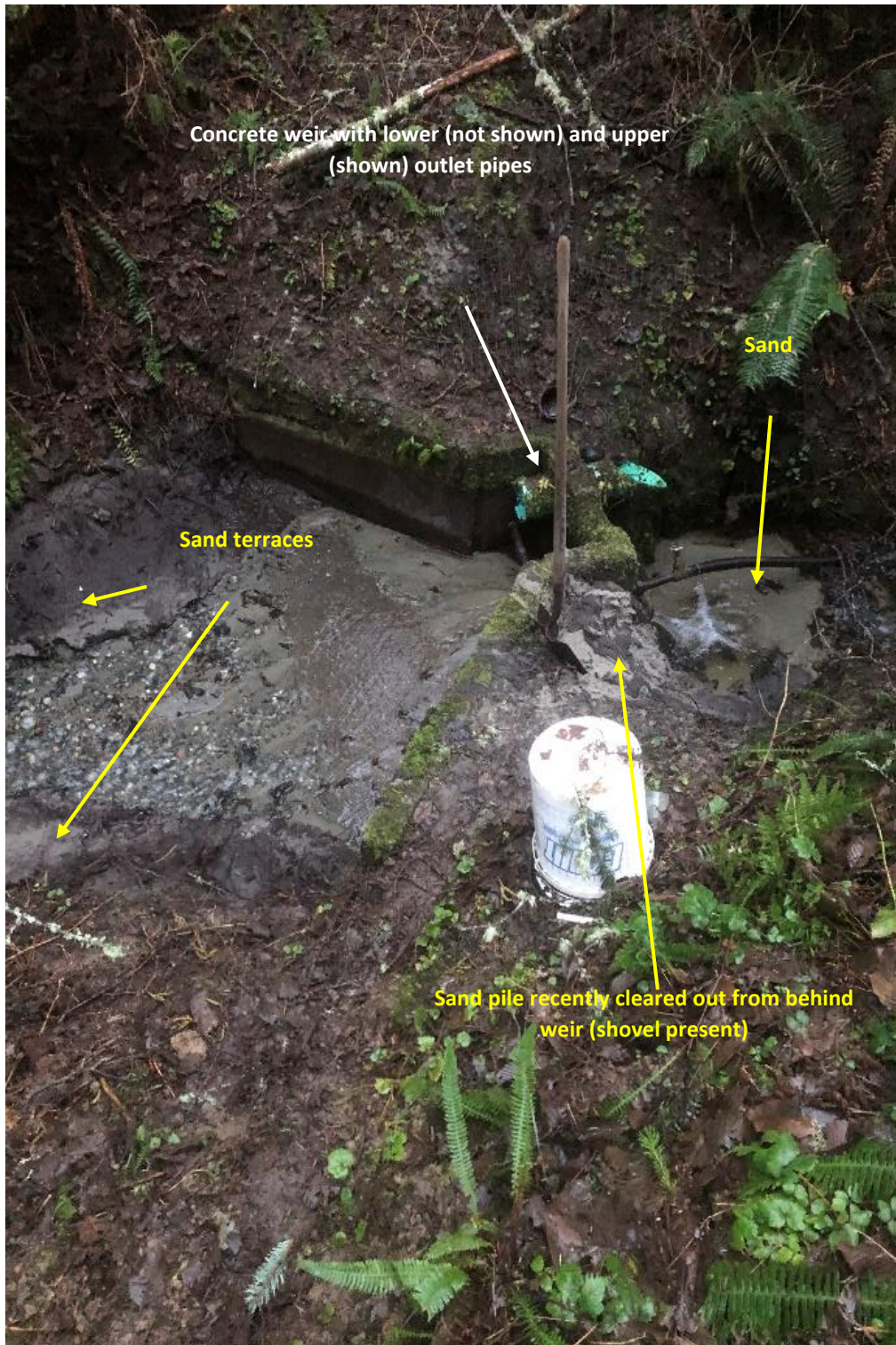
Photo 15: Small concrete weir near lower portions of drainage outlet that is maintained by the greenhouse operator. Note evidence indicates the operator needs to periodically clear out sand deposits from behind the weir.
