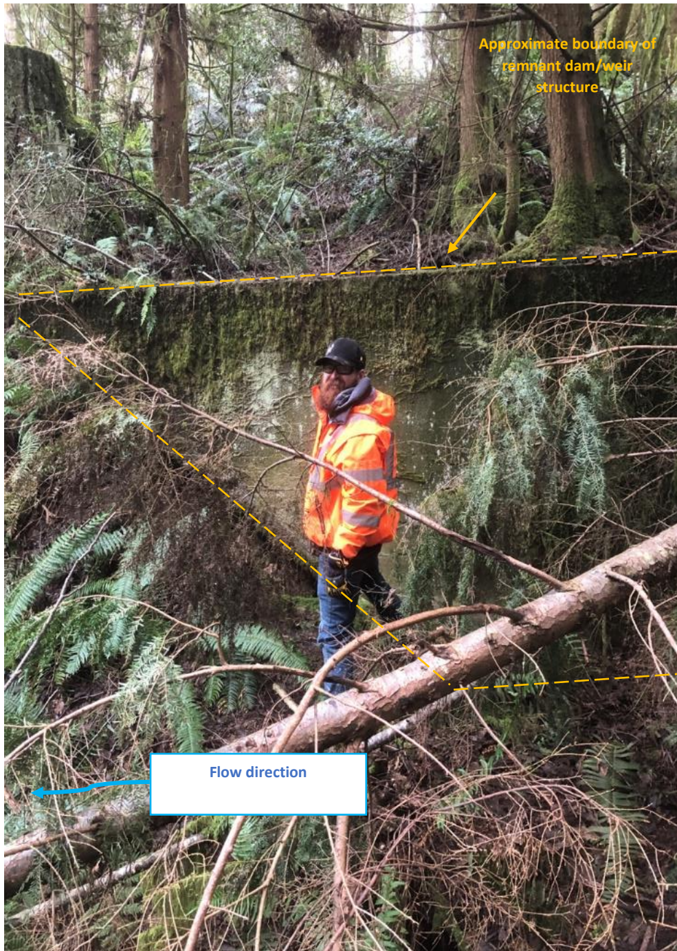
Photo 14: View facing south at the remnants of an abandoned concrete dam/weir located near the head of the drainage that outlets from the reservoir amphitheater. A corresponding structure is located on the north side of the channel behind the photographer. The dam/weir may have been used to pipe water to the Port Gamble mill site.
