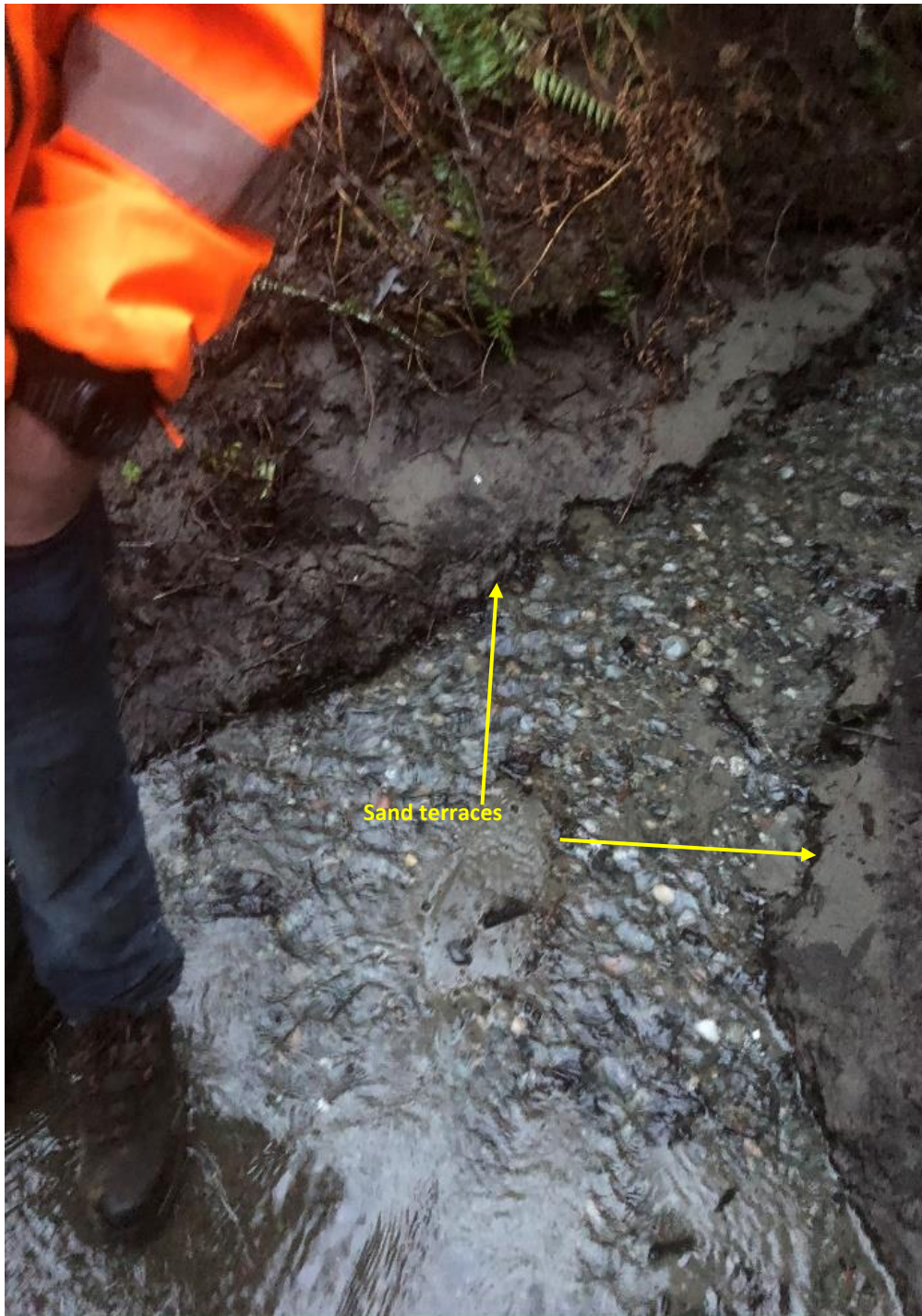
Photo 16: Sand terraces observed behind the small concrete weir indicate sand eroded from the reservoir amphitheater can accumulate behind the weir when not maintained regularly.
