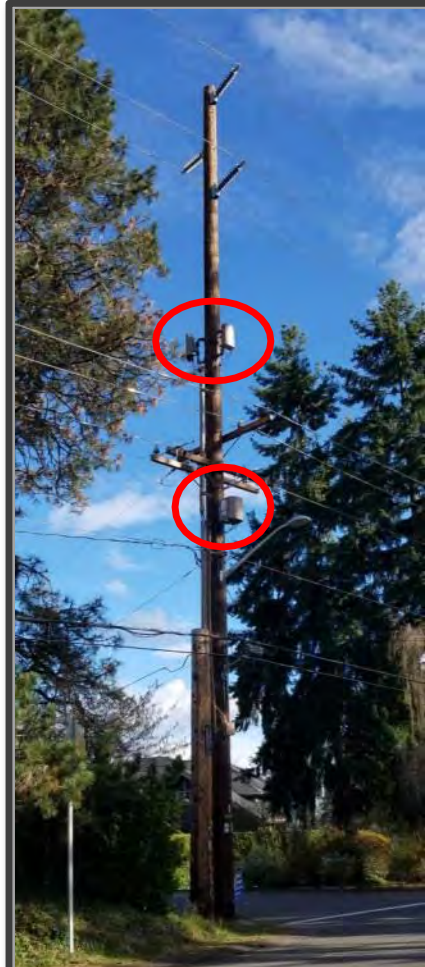
Small Cell on Utility Pole
