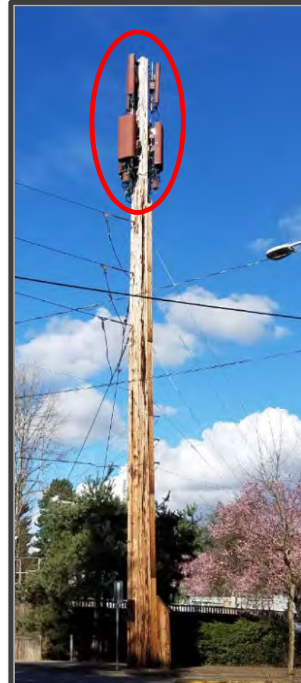
Macro Site on Utility Pole
