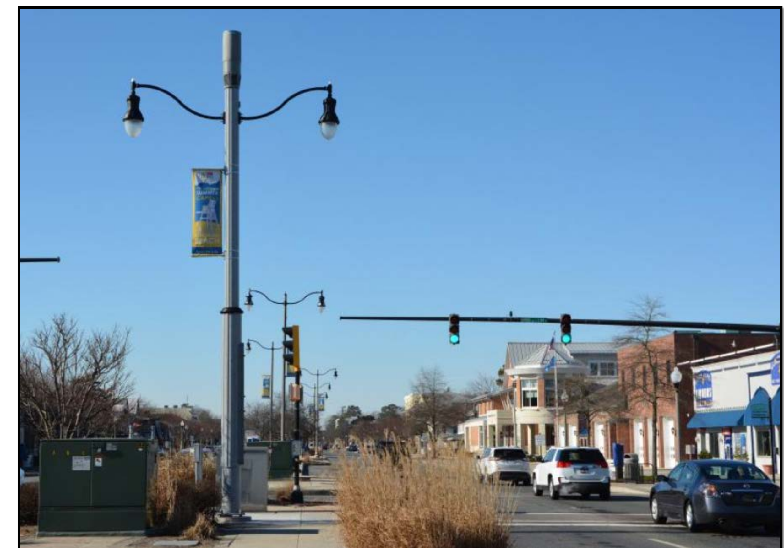
Image Source: https://www.capegazette.com/article/five-att-cellphone-towers-installed-rehoboth/171309#&gid=1&pid=4
