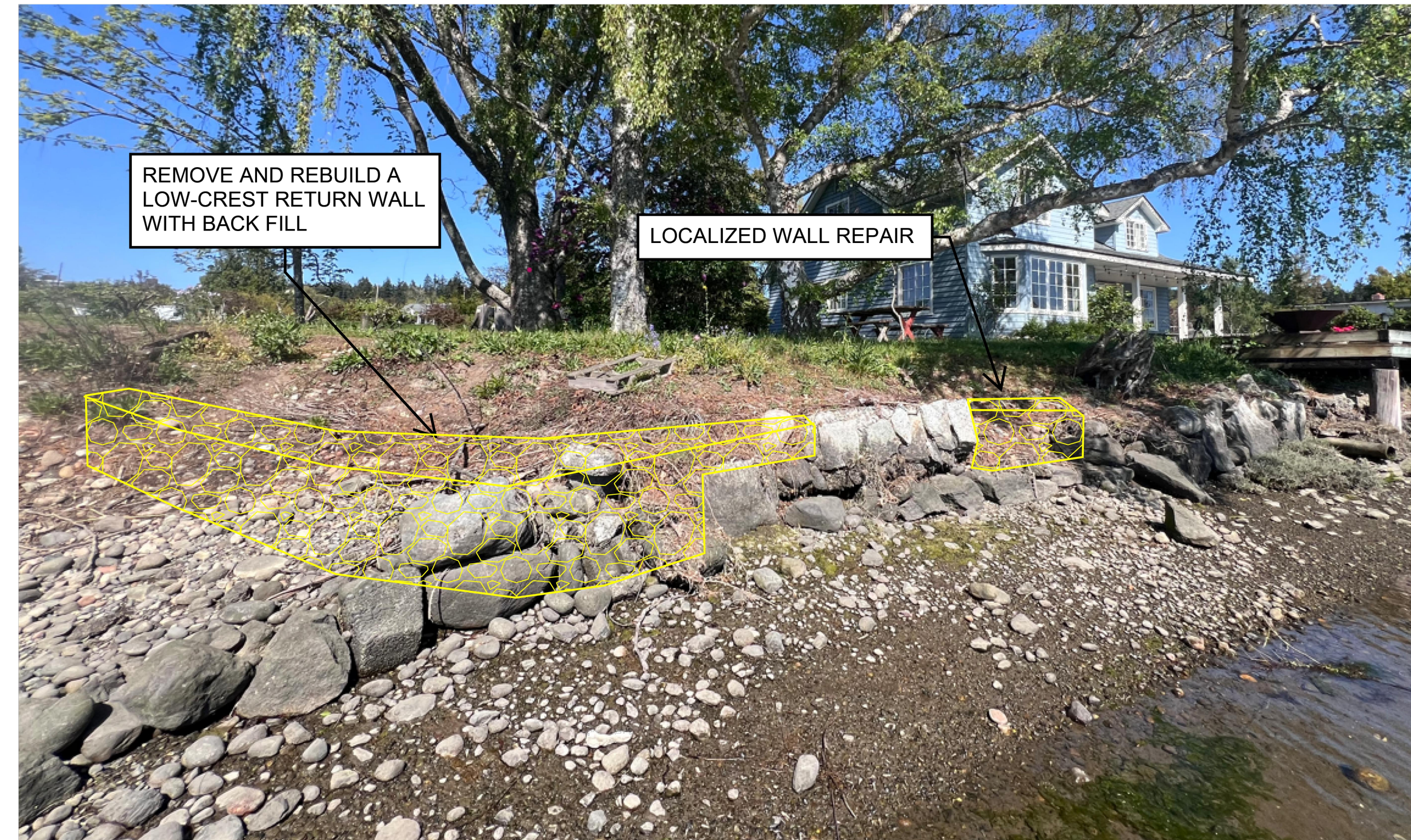
C ROCK RETURN WALL AT SECTION B (ILLUSTRATION ONLY, NOT TO SCALE)
