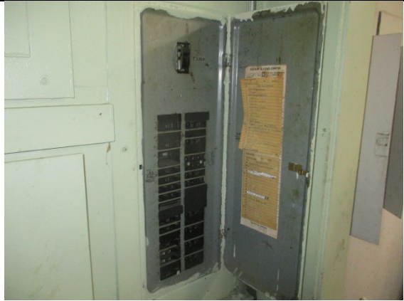
Upper-level power panel
