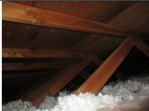
Old staining at attic area
