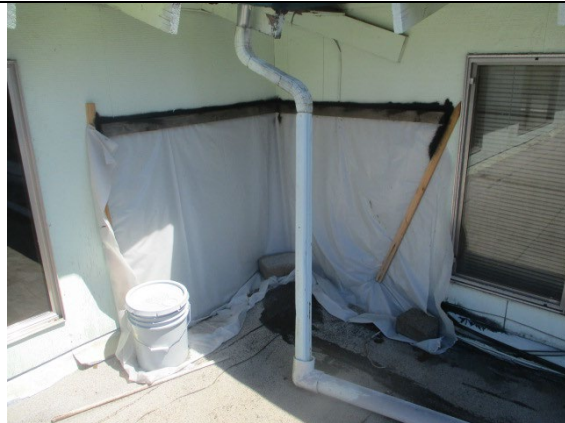
Upper northeast corner parapet that is not sealed or finished
