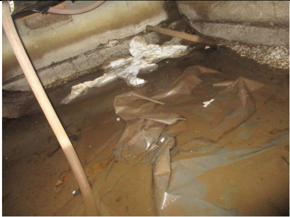
Water in crawlspace
