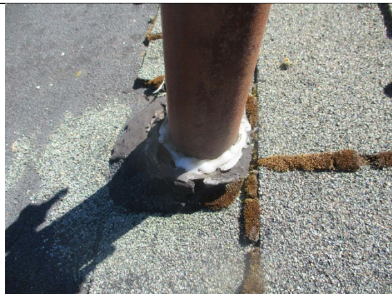
Deteriorated plumbing vent pipe boot that should be replaced
