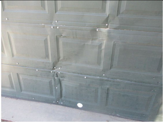
Damage at south overhead door
