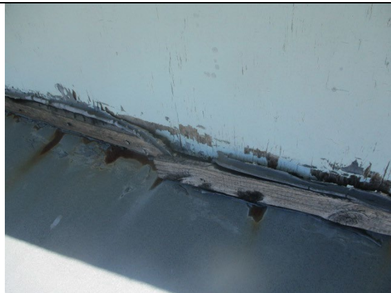
Gap in flashing at gable wall
