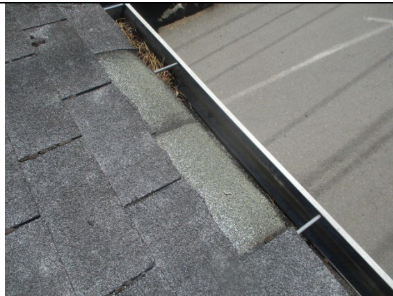
Missing roofing at the gutter line at cart storage
