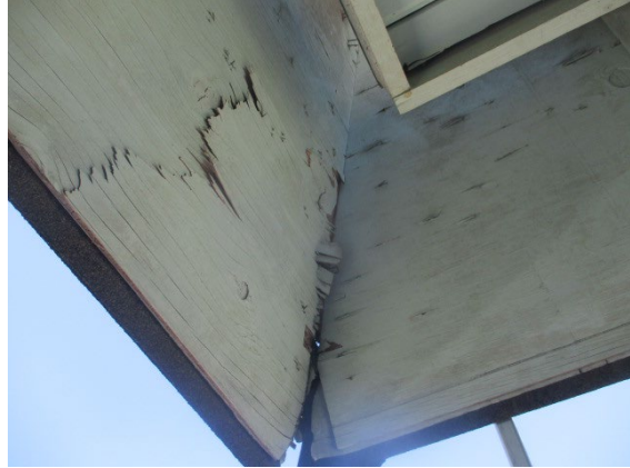
Damage at northwest corner of entry roof from vehicle, contact
