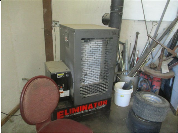
Oil fueled heater
