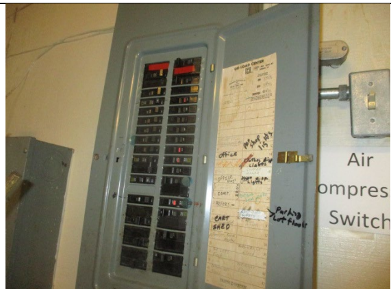
Pro shop power panel
