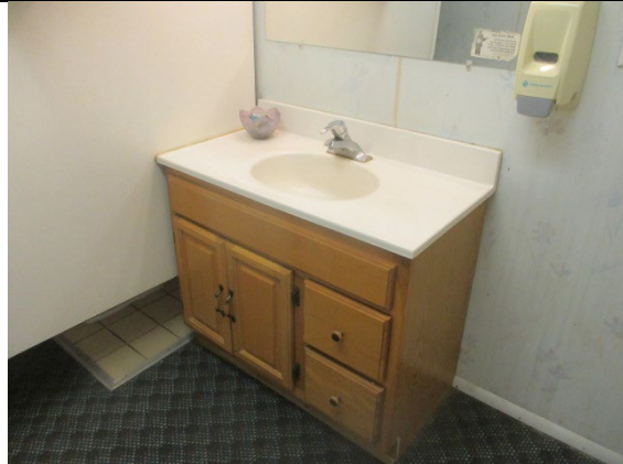
Typical vanity that is not ADA compliant
