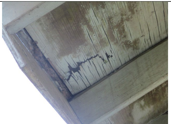
Damage sheathing at mansard
