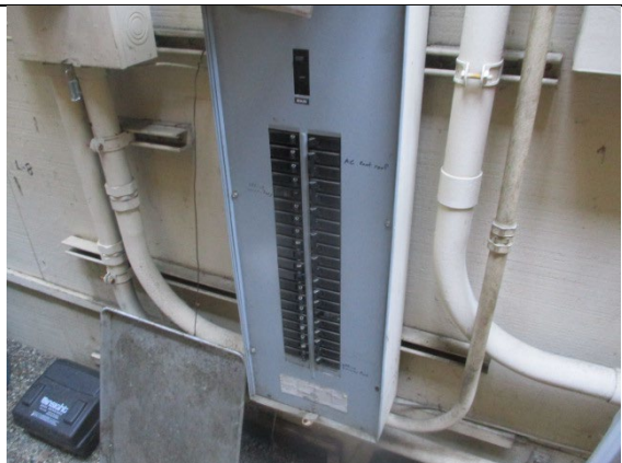
Exterior power panel on the north side
