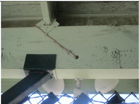
Exposed electrical wires at cart storage
