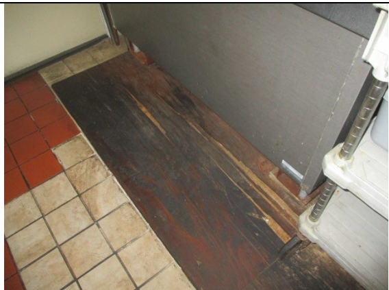
Missing flooring and extensive wood decay under icemaker at kitchen
