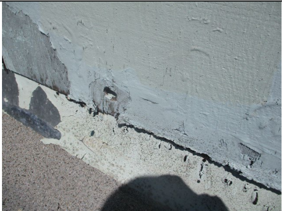
Damage siding and loose flashing at parapet
