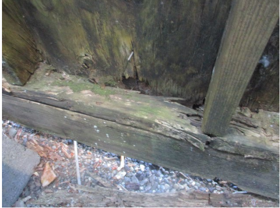
Wood decay in the sill plate and siding at north screen wall
