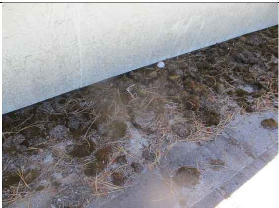
Deteriorated roof at breezeway
