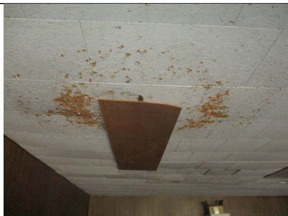
Older staining at upper ceiling
