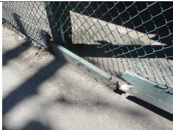
Damage screen at east side of cart storage
