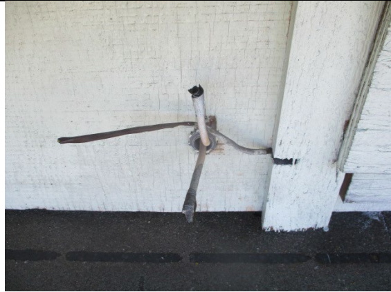
Exposed wires at gable end that should be placed inside of an approved junction box with a cover
