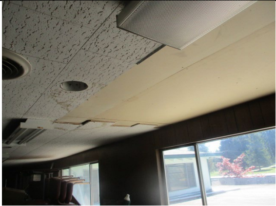
Missing ceiling tiles at the upper level
