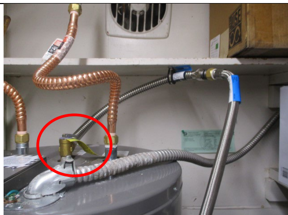
restaurant water heater missing thermal expansion tank and discharge line from temperature pressure relief valve
