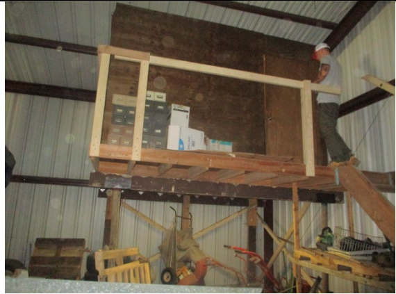
Loft without handrail on stairs
