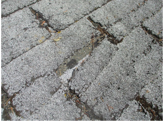
Deteriorated roofing at cart storage
