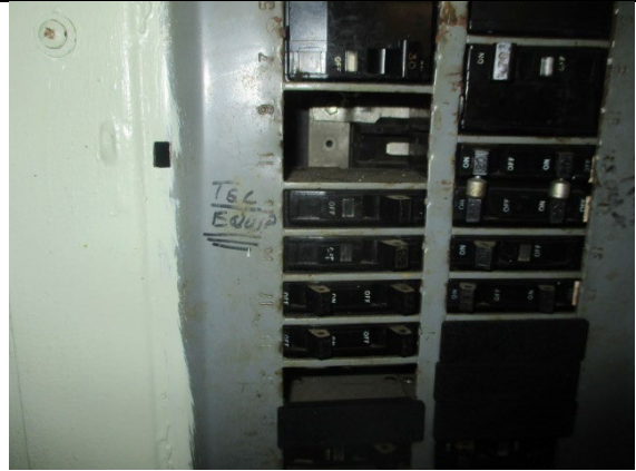
Kitchen power panel
