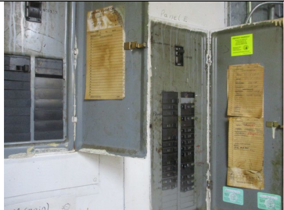
Kitchen power panels
