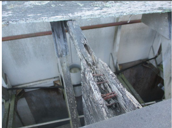
Wood decay in framing at screen wall
