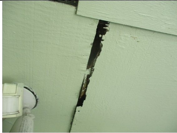
Loose soffit at southwest corner of restaurant
