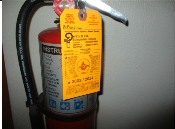
expired fire extinguisher service date
