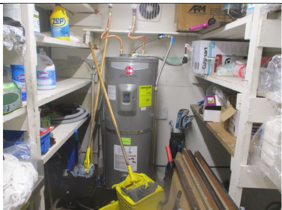
Restaurant water heater with a single seismic restraint strap and no thermal expansion tank or discharge line from temperature and pressure relief valve
