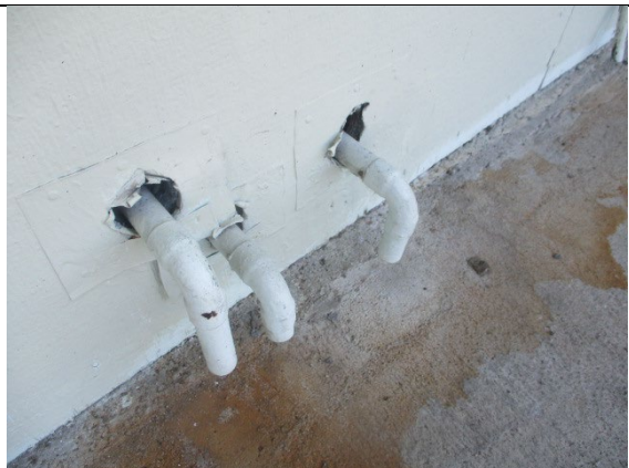
Westside lines need to be caulked and sealed at siding
