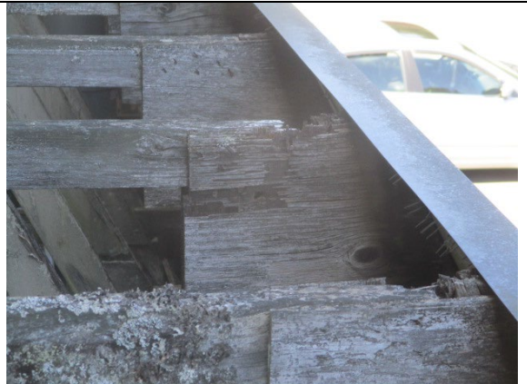
Wood decay in framing at screen wall and north side
