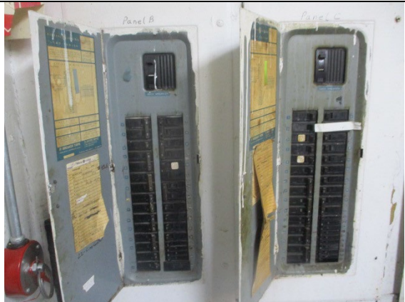
Kitchen power panels
