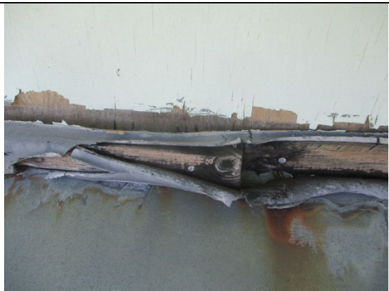
Gap in flashing at parapet wall
