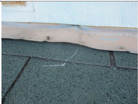
Loose flashing at the gable end
