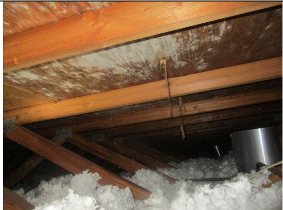
Staining at roof sheathing in attic
