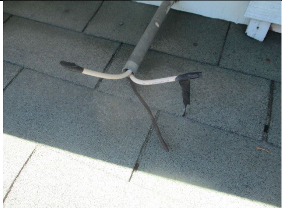
Typical exposed wires at Gable end that need to be capped off in a junction box
