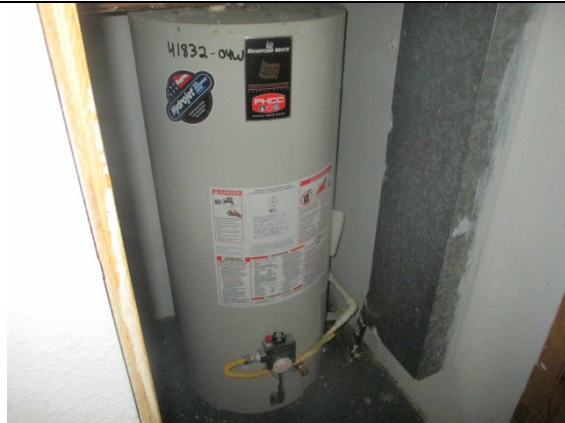
Upper-level gas water heater without seismic restraint straps and no thermal expansion tank
