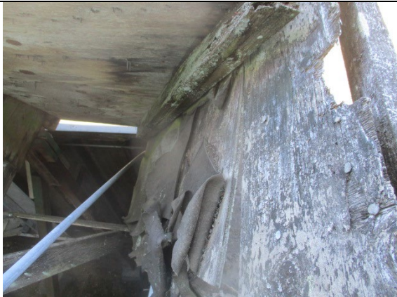
Wood decay in top of screen wall at Northside
