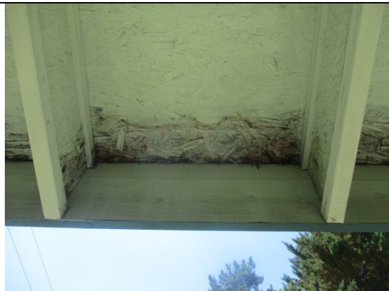
Wood decay in the soffit at cart storage
