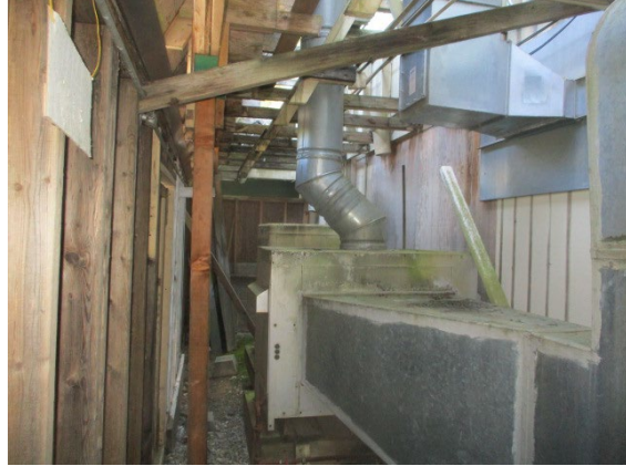
Area at north screen wall with HVAC equipment
