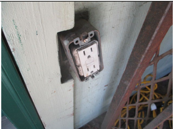
Electrical outlets at storage area that needs weatherproof cover.
