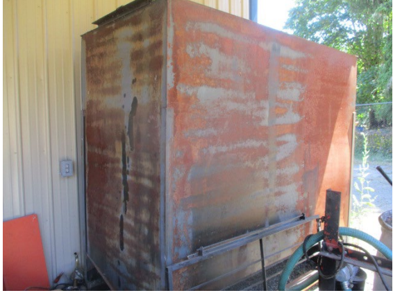
Above ground fuel oil storage tank
