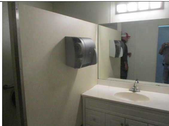
Typical restroom dispenser that is over 40 inches above the floor and is not ADA compliant
