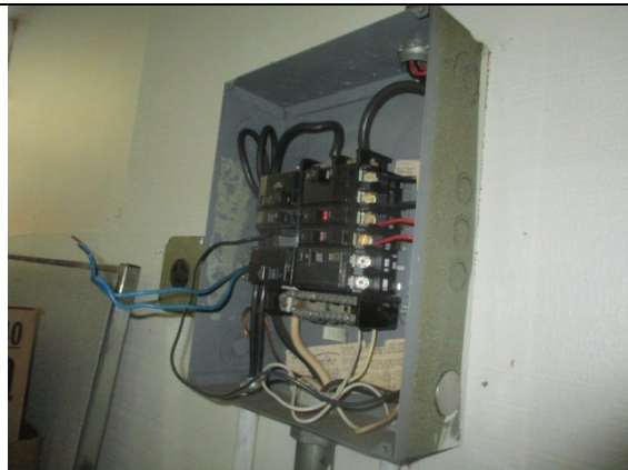
Open power panel at office above West End of restaurant
