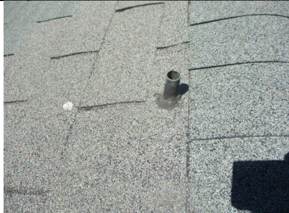
Plumbing vent at upper roof without a boot around it.
