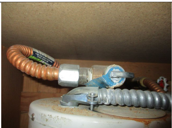
Upper bath water heater with temperature and pressure relief valve that runs uphill
