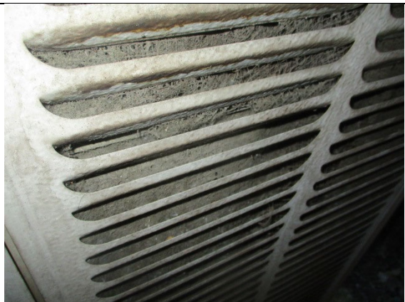
Plug vent at older HVAC unit on the north side
