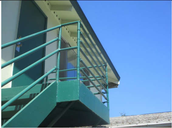
Open railing at east stairway
