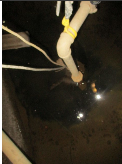
Sump pump at crawlspace
