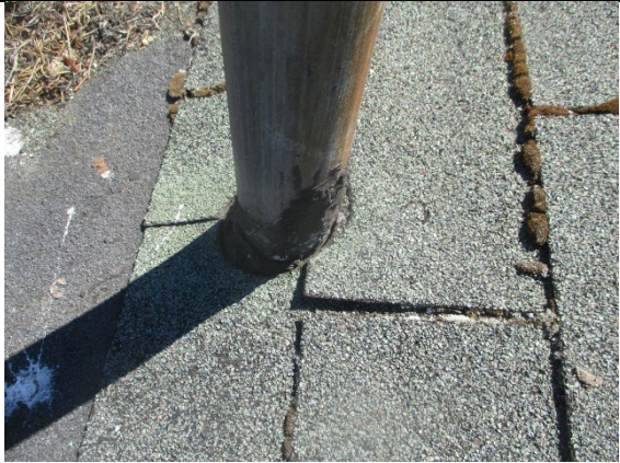
Plumbing vent pipe the needs to have a boot installed that is above the roofing to drain properly
