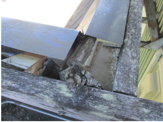
Gap in flashing above entry
