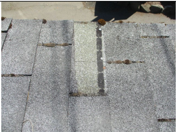
Missing roofing at cart storage
