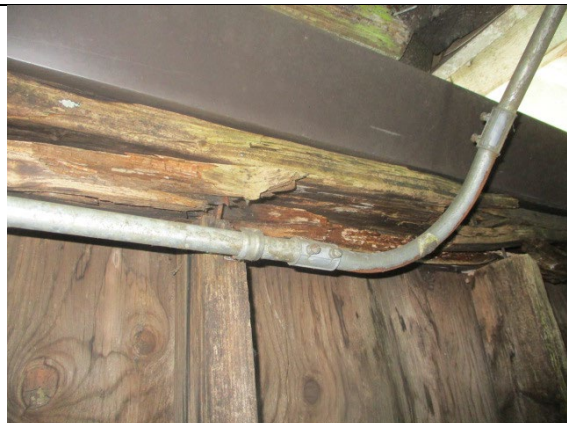
Wood decay in top plate at screen wall on the north side
