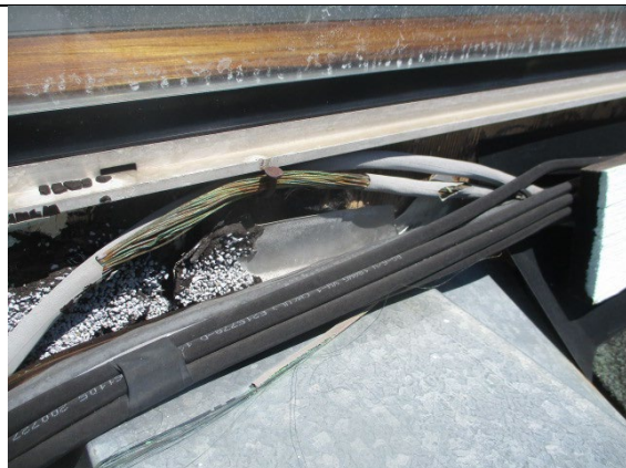
Exposed wires at parapet that need to be sealed/protected
