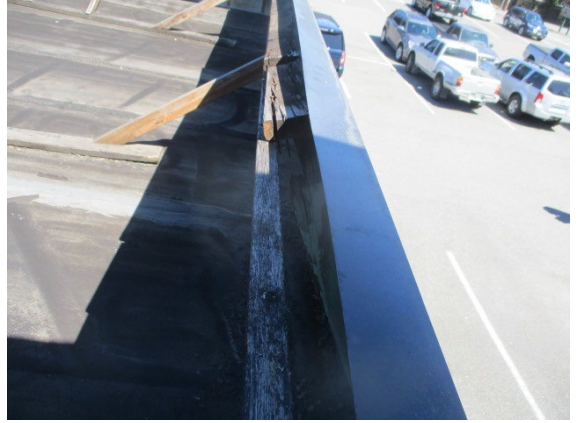
Loose flashing and some wood decay at top of screen wall on the north side
