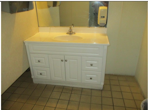
Typical the vanity that is not the compliant as it is closed on the area under the sink
