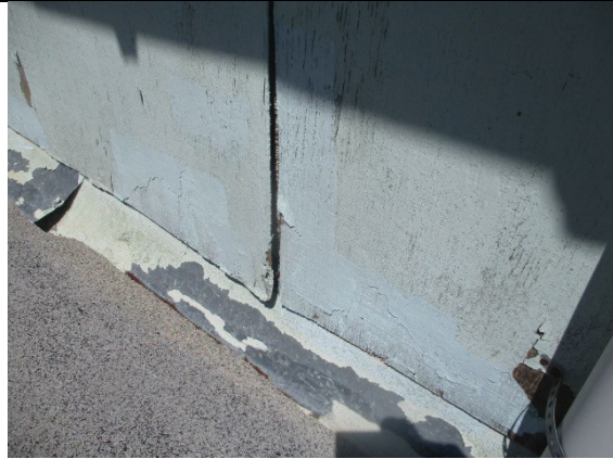
Loose siding and flashing at parapet above restaurant
