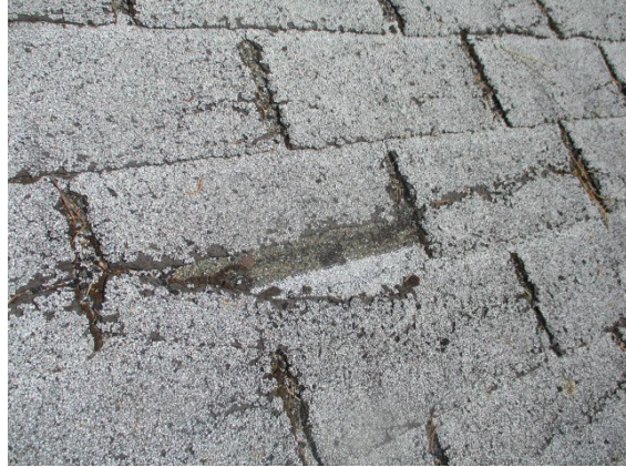
Deteriorated roofing at cart storage
