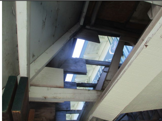
Open soffit area along the north side
