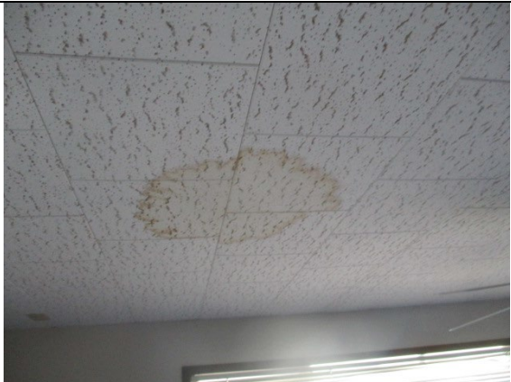
Stains from old roof leak
