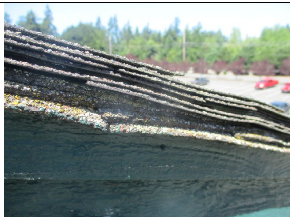
Multiple layers of roofing at cart storage area
