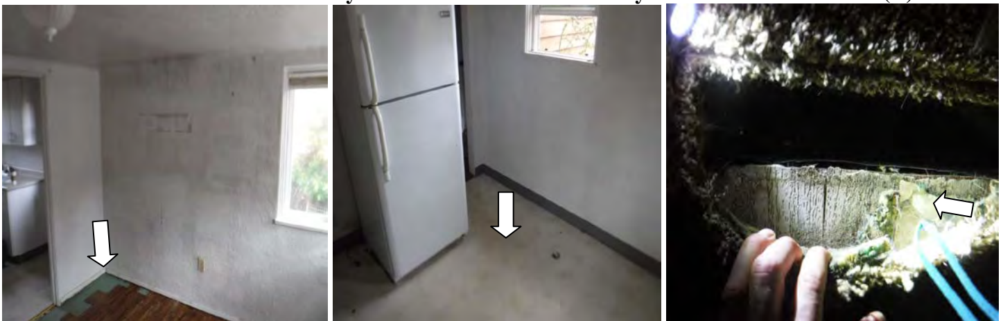
Photos 1-3: Representative Photos of Green Sheet Vinyl (Under Vinyl Plank Flooring) in Living Room (L), White Sheet Vinyl over Plywood and Concealed Green Sheet Vinyl in Kitchen (C), and White “Wood-Patterned Sheet Vinyl in SW Bedroom and Hallway on Main Floor of House (R):
